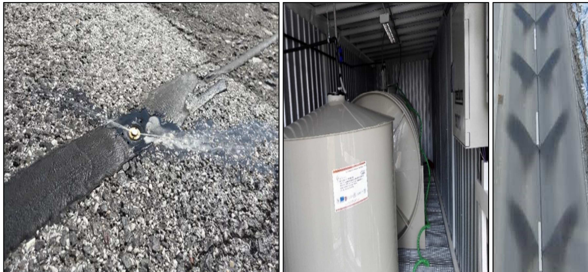
Figure 5. Automatized anti-icing spraying systems of University of Zilina. Source: authors' photos
